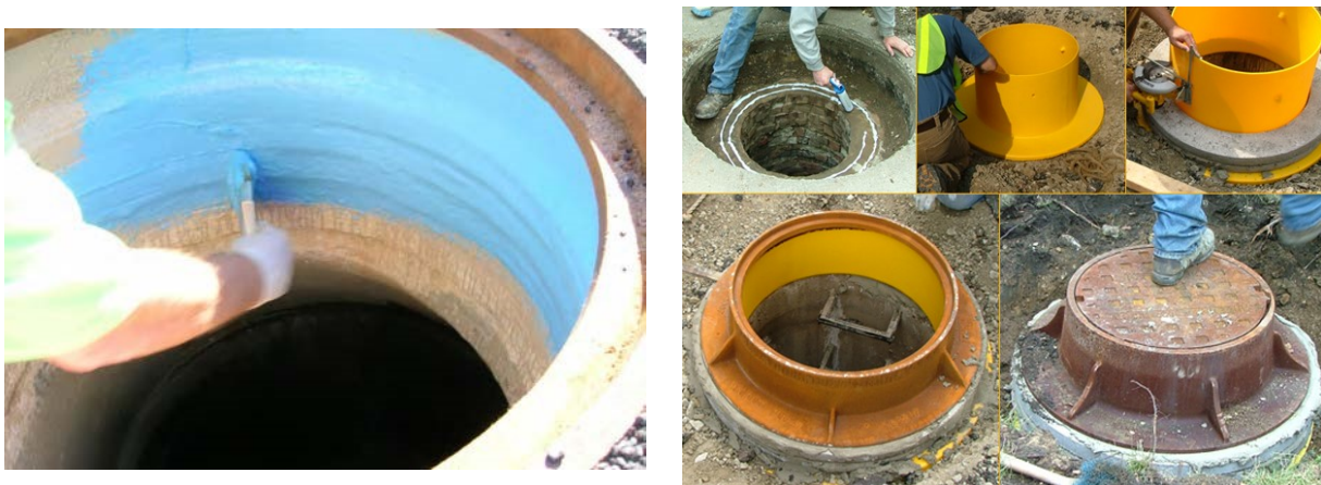
Figure 23. (a) application of Flex Seal Utility Sealant; (b) installation of I&I Barrier.
