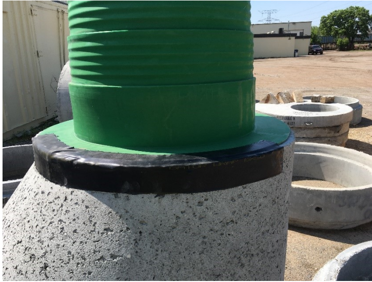
Figure 15. Alignment Barrier on cone with Gator Wrap placed around part of the flange.
