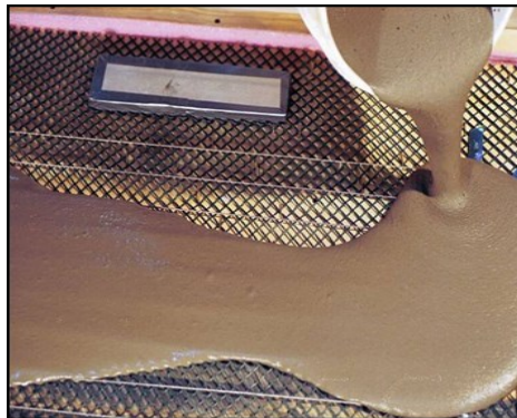
Applying Self-Leveling Floor Underlayment Cement on top of Plastic Lath with radiant heat cables
